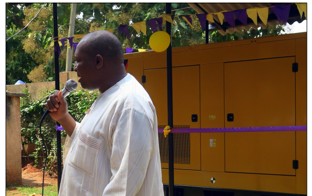
Rev. Emile Adoté, general superintendent of the AG-Benin and vice president of the Board of Governors, dedicates the new generator to God's service.
